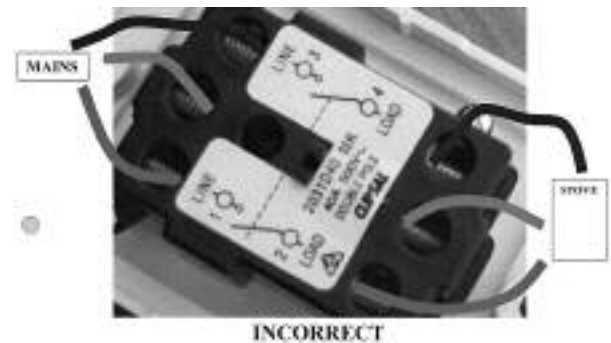
This is how the switch was incorrectly connected
