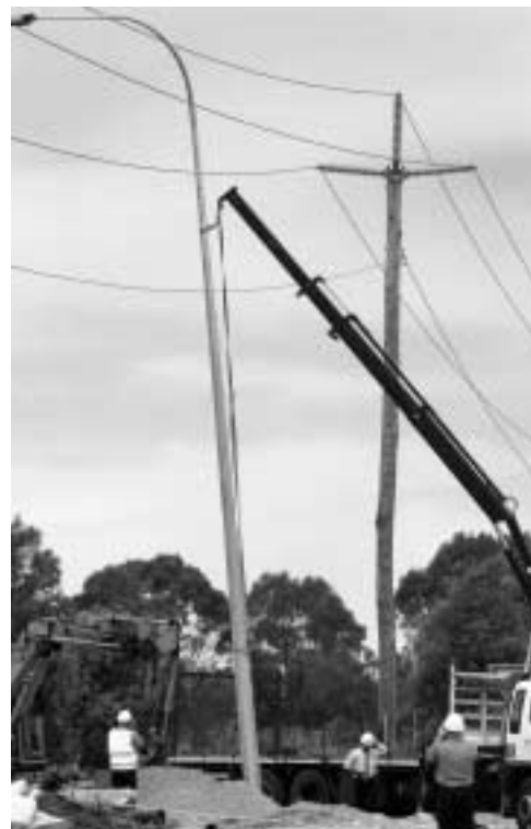
This streetlight column contacted 132 kV power lines
