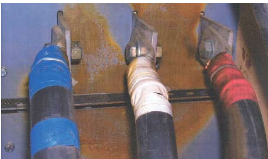
Area of flashover at the rear of the CFS unit
