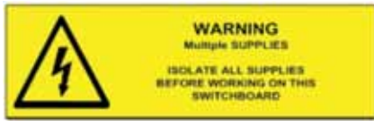
Figure 2: Typical warning label
