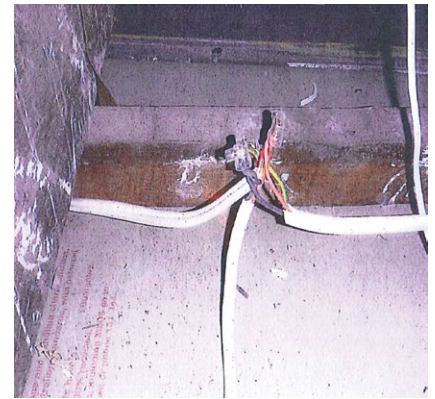
Unenclosed junctions found in the ceiling space
