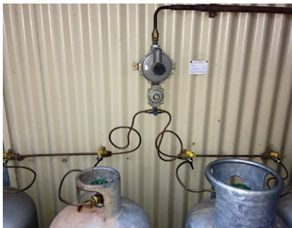
Fitzroy Crossing where a regulator was incorrectly installed upside down
