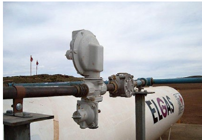
Mining camp in Pilbara with the incorrect regulator and filter fitted
