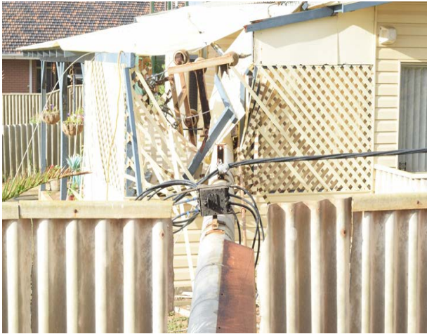
Fallen pole and conductors causing damage to the fence and patio
