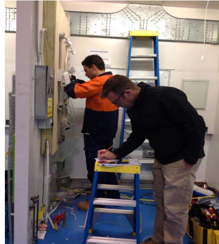
Chief Judge Todd Bell monitoring the progress of electrical apprentice Jacob Harding
