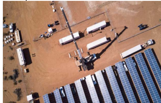
Aerial view of the solar array and BESS at site (Source: Carnegie Clean Energy)
