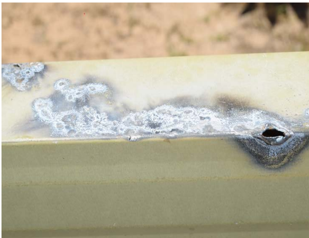
Burn marks on the fence cap
