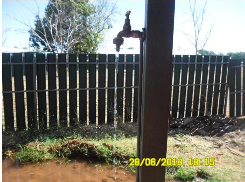
Bayulu Community Lot 34 Leaking Garden tap (replaced)
