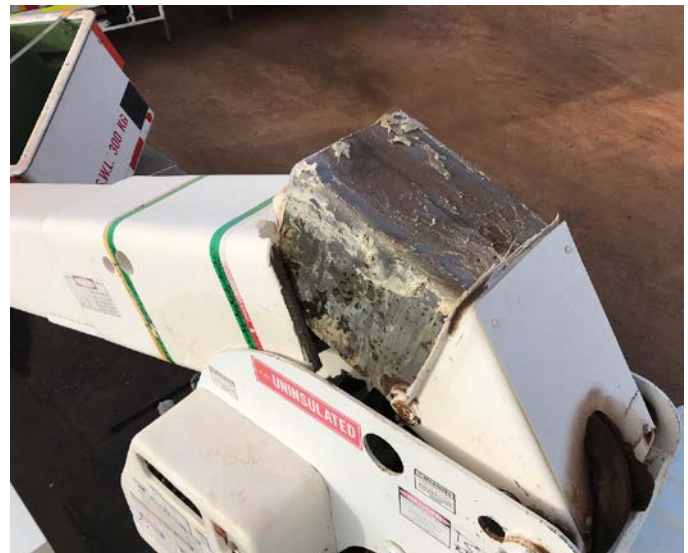
EWP boom failure between the metal support structure and fibreglass joint section.
