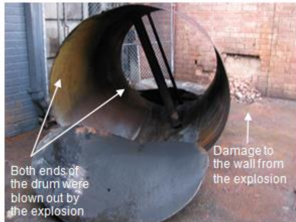
Image of the damaged drum and wall
