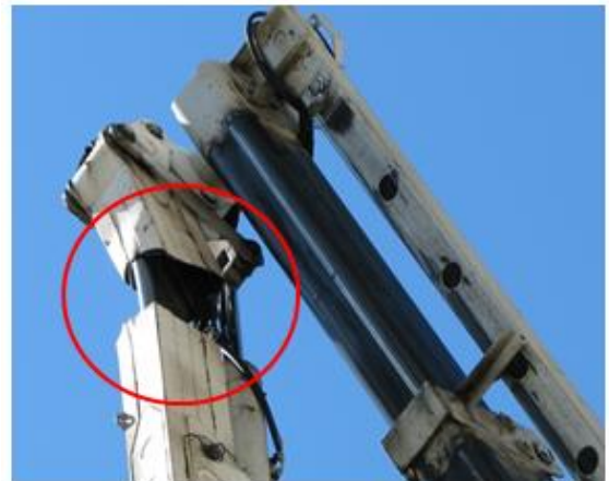
Figure 1 Area of jib failure
