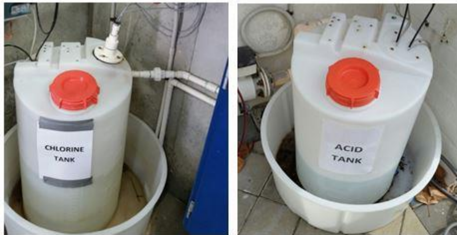
When the incident occurred these drums were not labelled and were almost identical in appearance. The photos show temporary labels applied after the incident.
