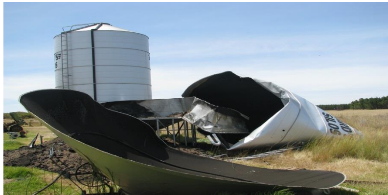
The explosion blew off the silo roof, and the remaining structure was demolished to access the fire
