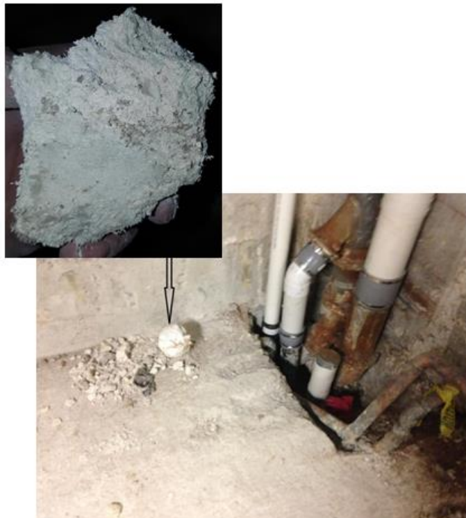
Work area showing asbestos-containing debris and close up of asbestos-containing debris
