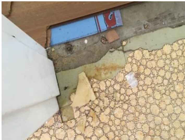
Asbestos vinyl tile under newer vinyl tile.
