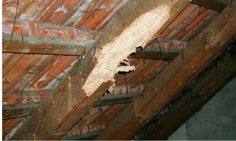
Structural pine broken away to expose EHB infestation.
