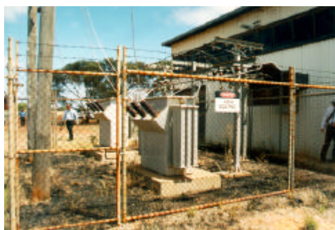
Transformer compound at Ladyloch Pumping Station
