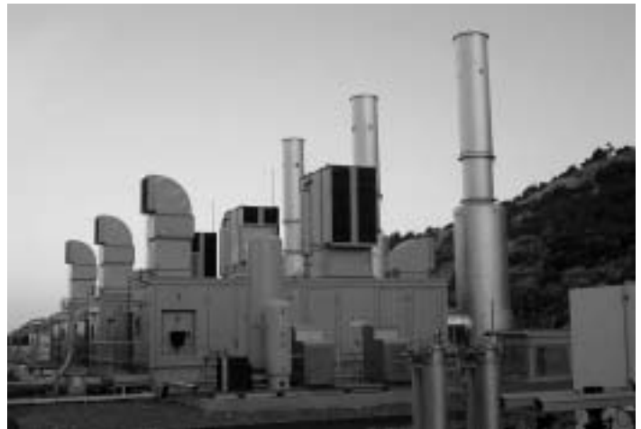
Esperance gas-fired power station
