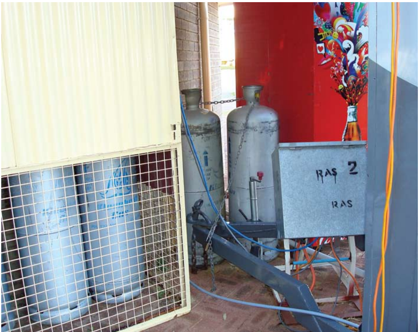
Non compliance: Gas bottles in prohibited zone near electrical meter box
