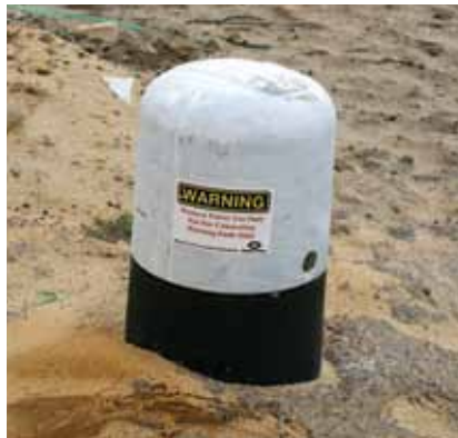
Photograph showing a working end pillar as how it should appear.
