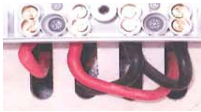
Photograph showing the transposed active and neutral conductors.
