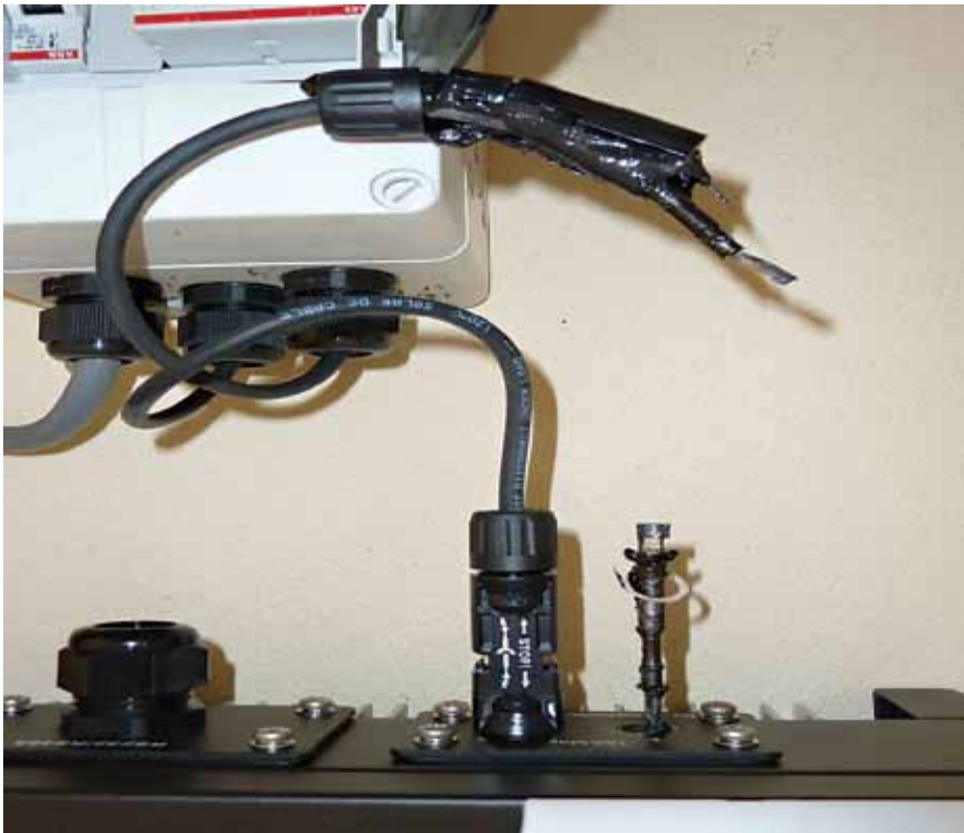
DC solar connector that has melted due to incorrect crimp termination.
