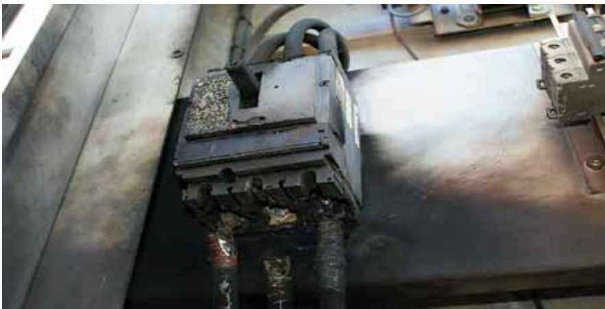
Damage caused to the switchboard from the earth fault.
