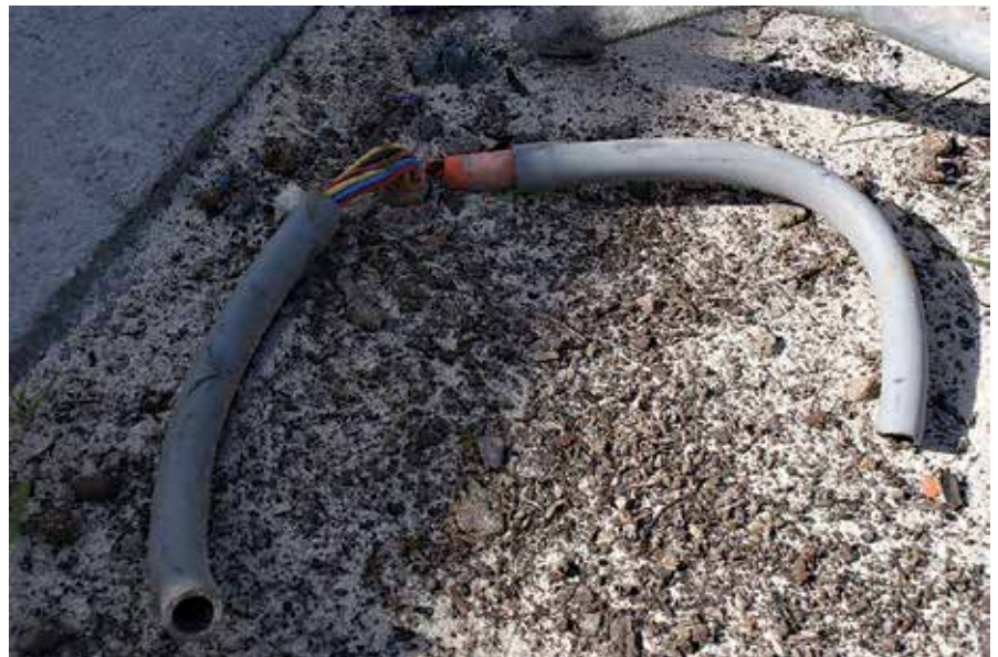
Photograph: Exposed cables discovered at an electrical installation on Rottnest.
