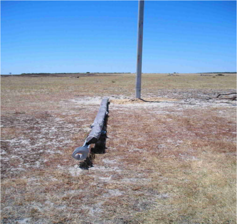
Photograph of Fire Scene with the Replacement Steel Pole and Failed Wooden Pole (D577/4 east)
