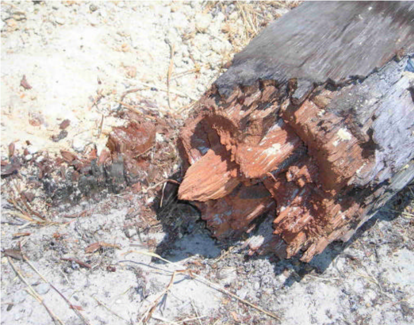
Photograph of the Failed Wooden Pole (D577/4 east)
