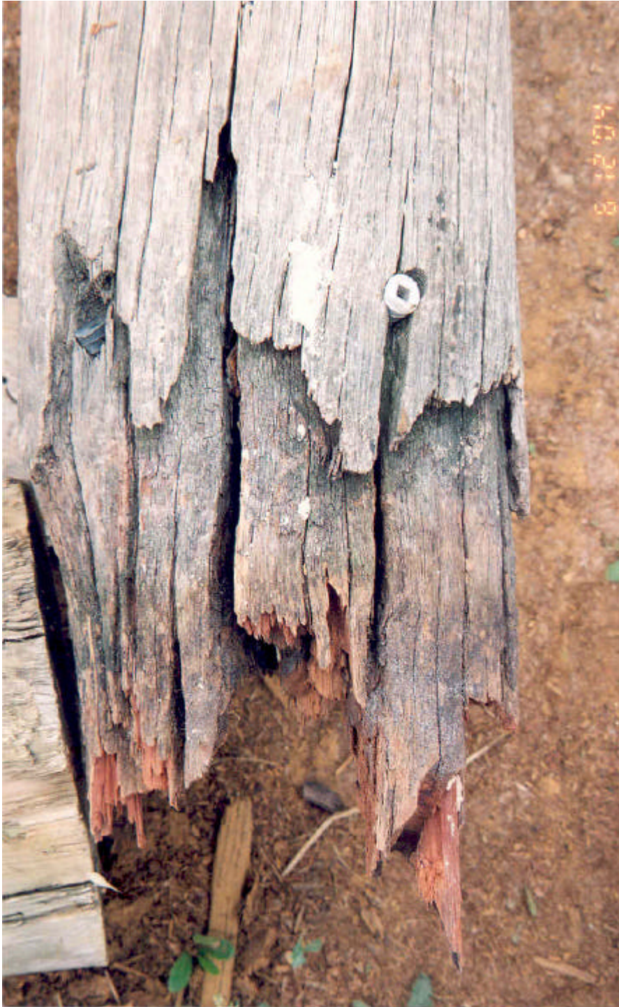
Photograph of Broken End of Pole D595/8 South
