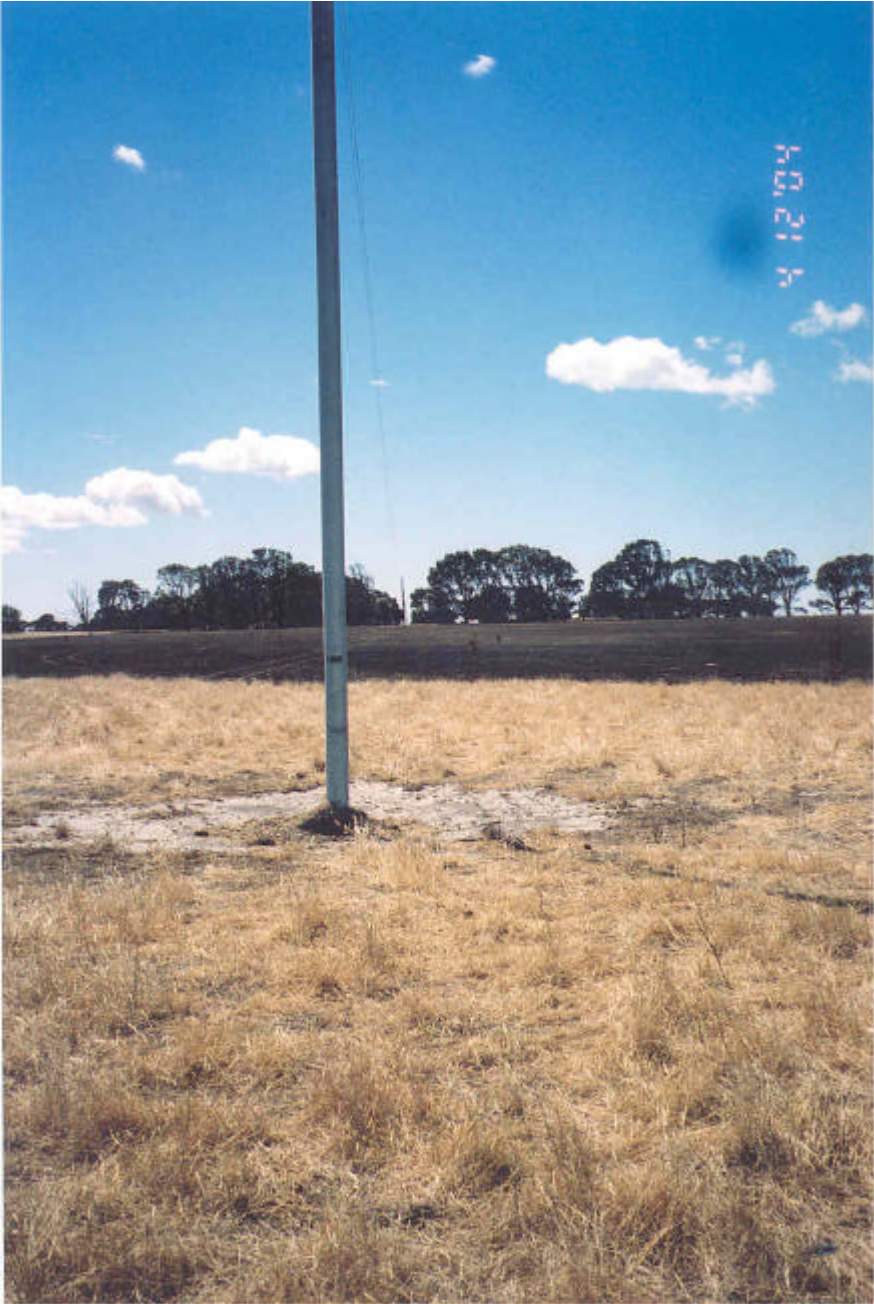
Photograph of Fire Scene with the New Replacement Steel Pole (D595/8 south)
