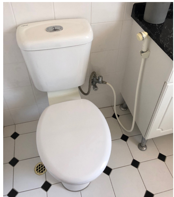
Photo 1: Example of a non-compliant installation
