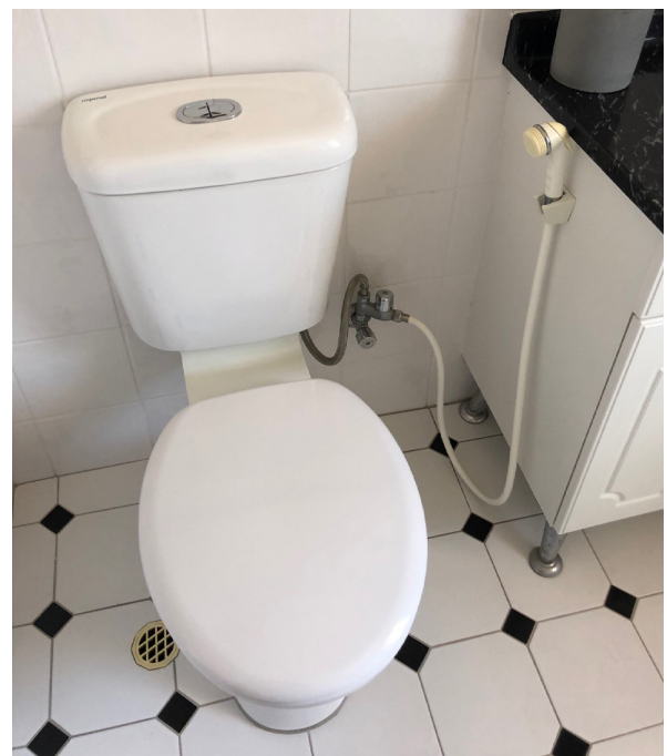
Photo 1: Example of a non-compliant installation
