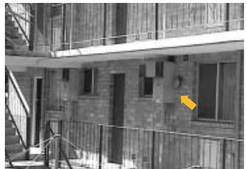
Typical installation that will require an exemption from the Director of Energy Safety before a changeover can be carried out
