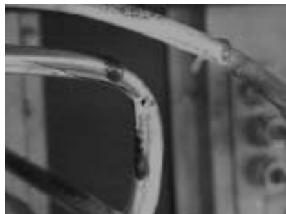
Drill damage to the aluminium tubing
