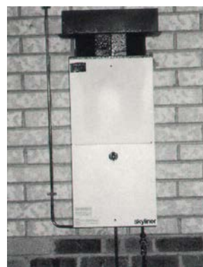
The relocated appliance shows heat damage to the casing and flue terminal
