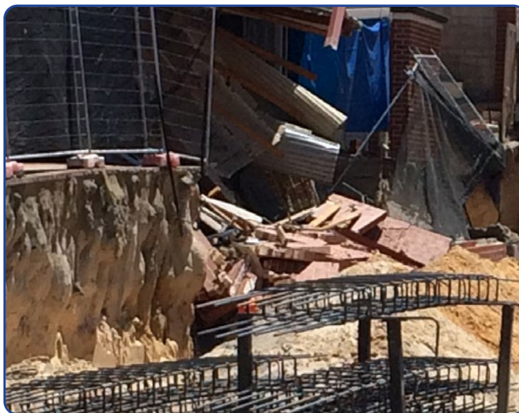
Figure 2: Insufficient and undermined grout injection works may result in undermining of land and structures
