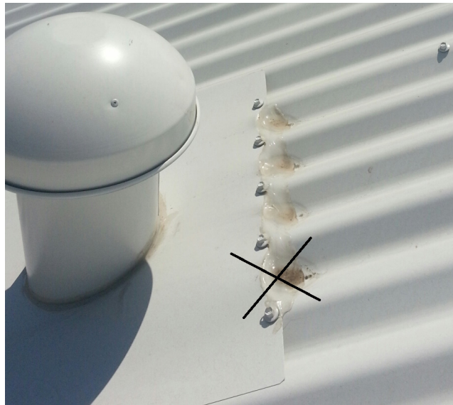
Flue tray not adequately flashed to prevent water penetration and inadequate provision made for drainage.
