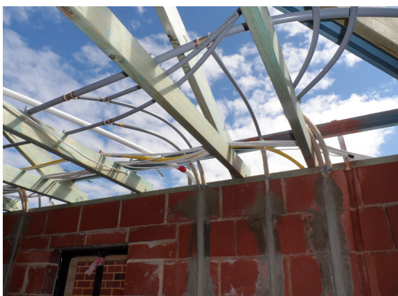
Photo 1: Minimum of 25mm separation required between cold water services, gas pipes and electrical cables. 100mm minimum separation required between heated water services, gas pipes and electrical cables.
