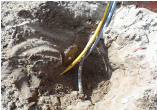
Photo 3: Minimum 600mm separation required between water services (grey pipe) and gas (yellow pipe), because there is no indicator tape or mechanical protection to the gas service.
