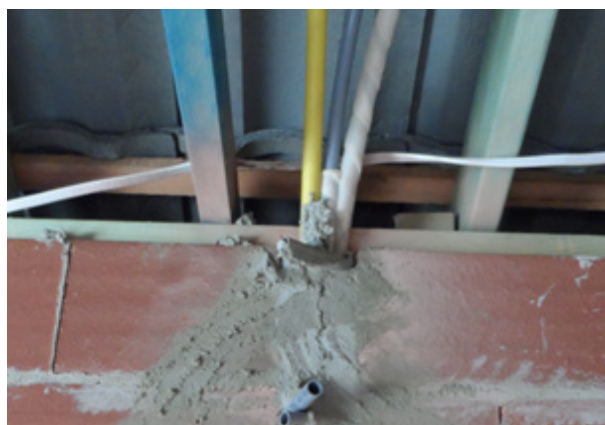
Photo 2: Minimum 100mm separation required between the heated water service (middle grey pipe) and gas (yellow pipe). Minimum separation of 100mm is required between heated water service pipe and electrical cables. Minimum 25mm separation between the electrical cable and the gas service pipes.
