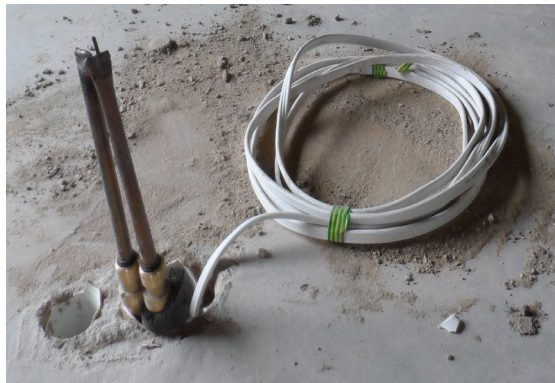
Photo 4: Minimum 100mm separation required between water services and electrical cable.
