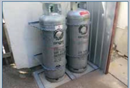
Cylinders chained to support structure
