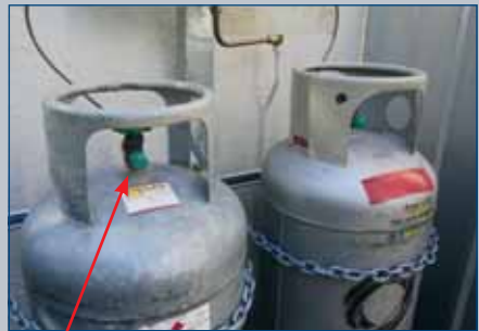
Safety valve discharge is protected by a plastic cap.
