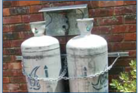
Cylinders chained to support structure
