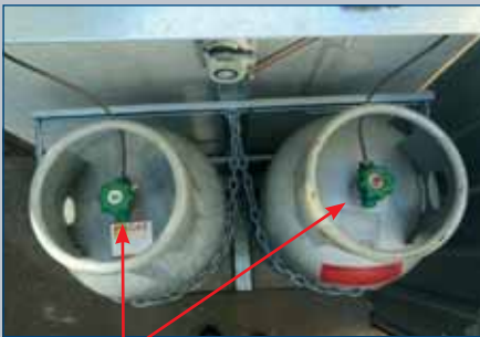
Safety valves should point away from buildings and any adjacent cylinders.
