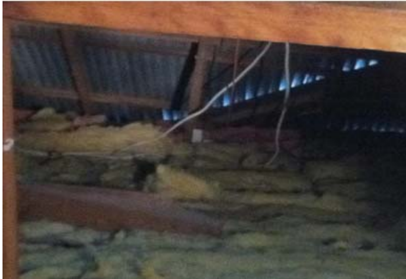
Figure 1: Typical case where cable is not properly secured
