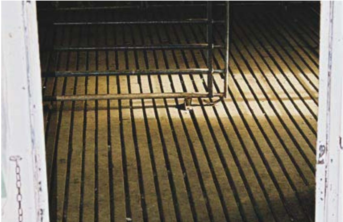
These battens in the catching pen are parallel to the direction of drag and are in good condition. Note: there is no light coming up through the boards.
