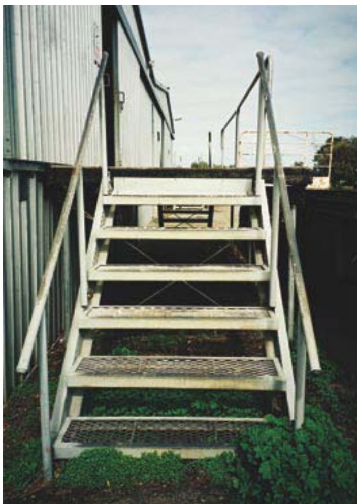
Safe access to the shed
