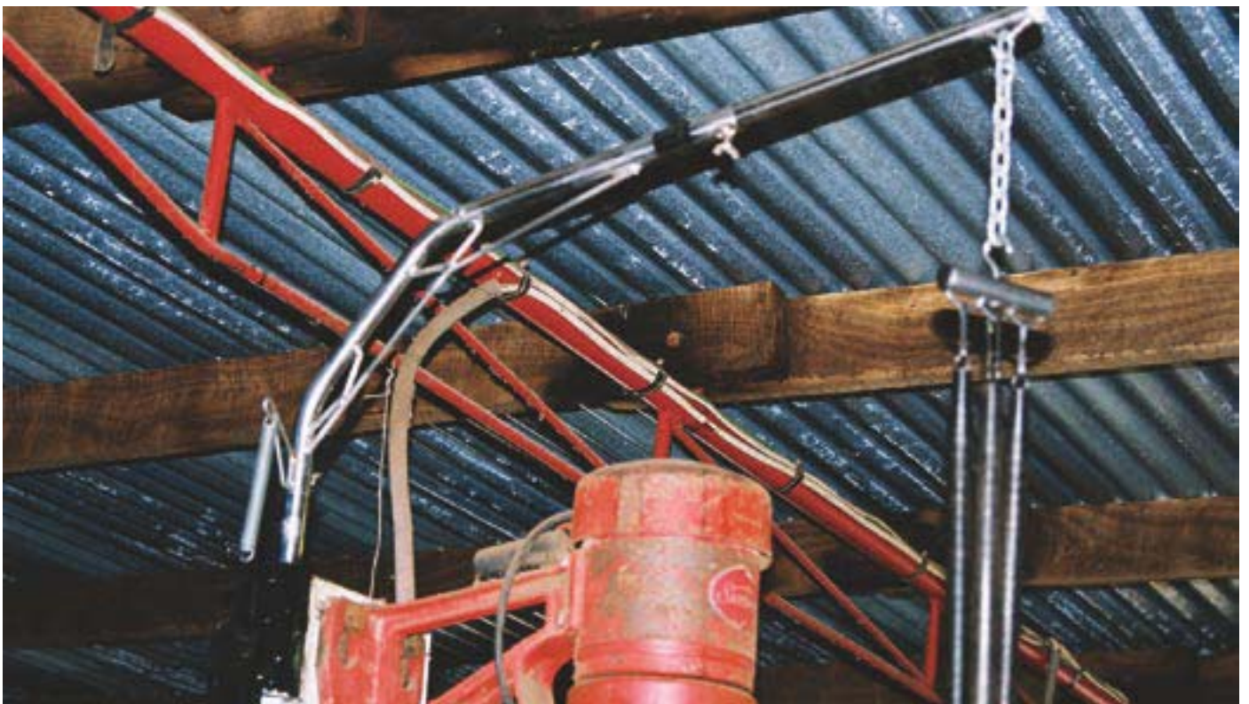
Cables kept well clear of the work area
