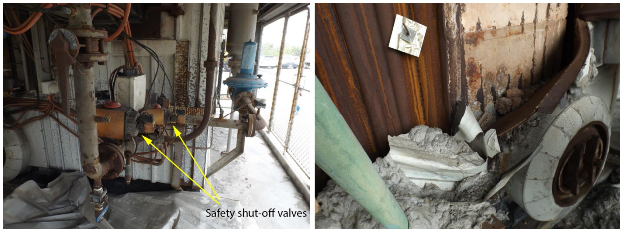
Left: Safety shut-off valves forming part of the burner management system. Right: Damage to boiler
