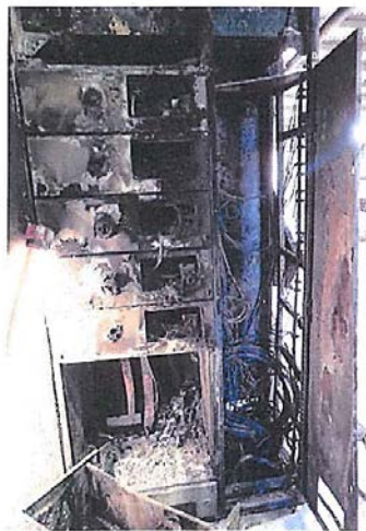
Damaged MCC modules
