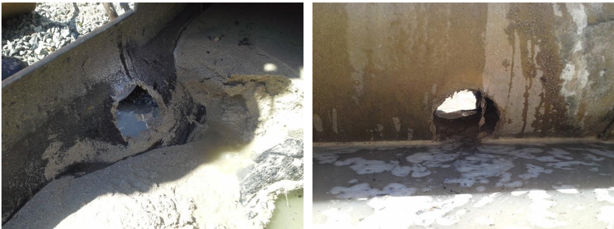
Damage to Water Corporation main sewer pipeline by underground horizontal directional drill Source Water Corporation
