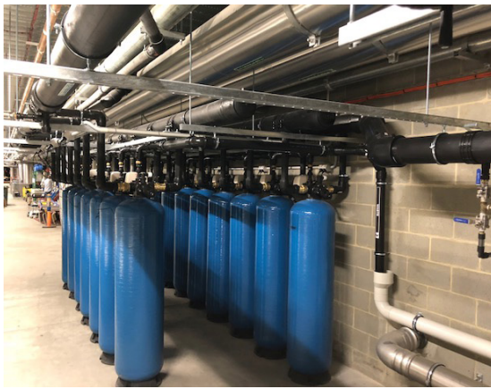
Photo 2: Commercial water filter installation
